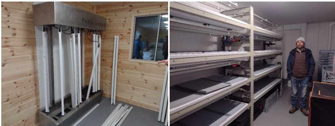
Figure 15: CEA equipment at the Treherbert pilot site
